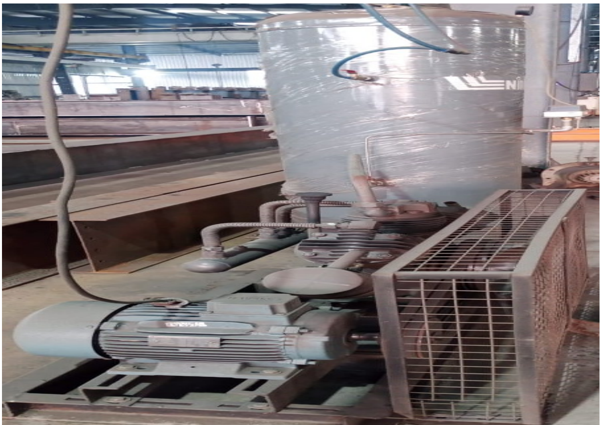
AIR COMPRESSORS (Capacity-7.5 Kg/Cm 2 )
