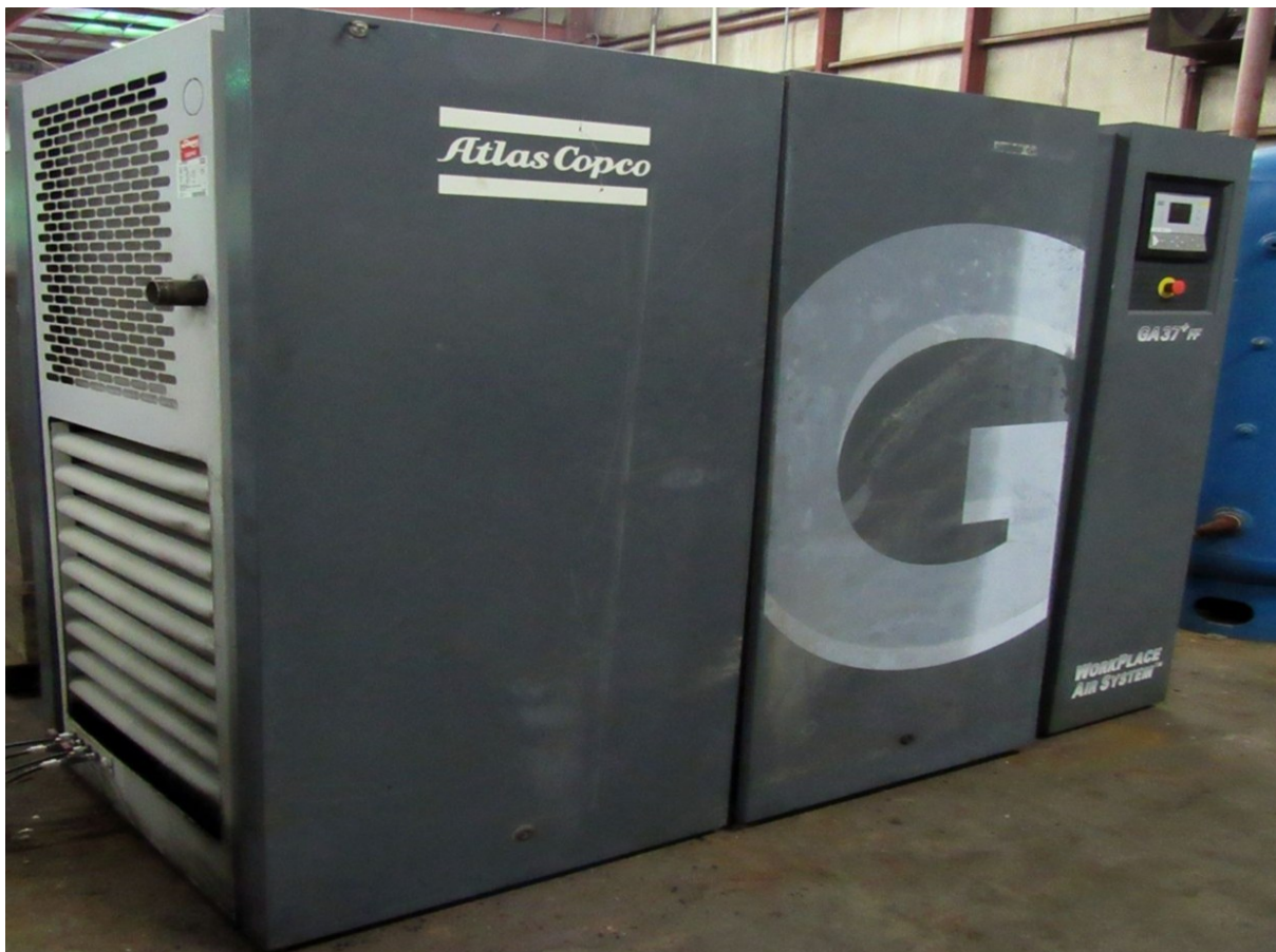
AIR COMPRESSORS (Capacity-7.5 Kg/Cm 2 )
