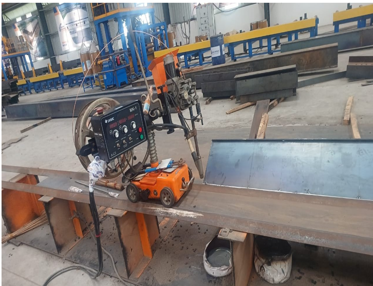
SEMI-AUTOMATIC SAW WELDING MACHINE
